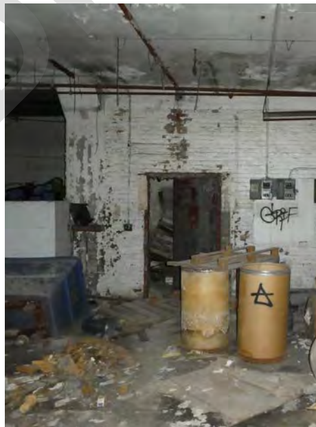
^ Debris and deterioration on the south building
